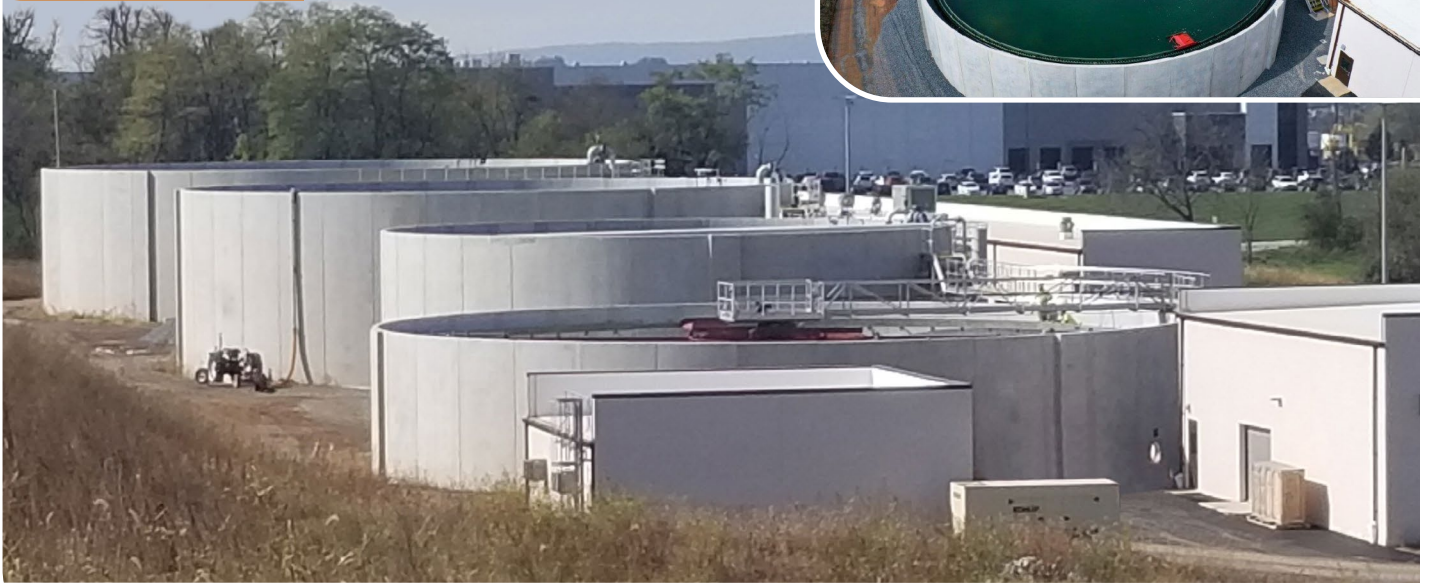
Treatment tanks with clarifier
