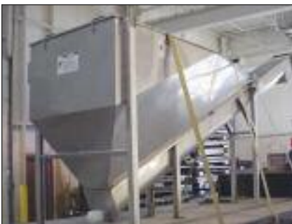
Installed Gritmeister unit
