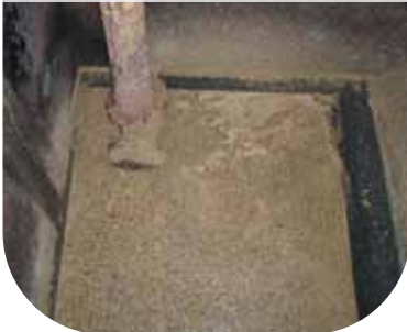
Ft. Collins, Colorado Before: 4" grease
