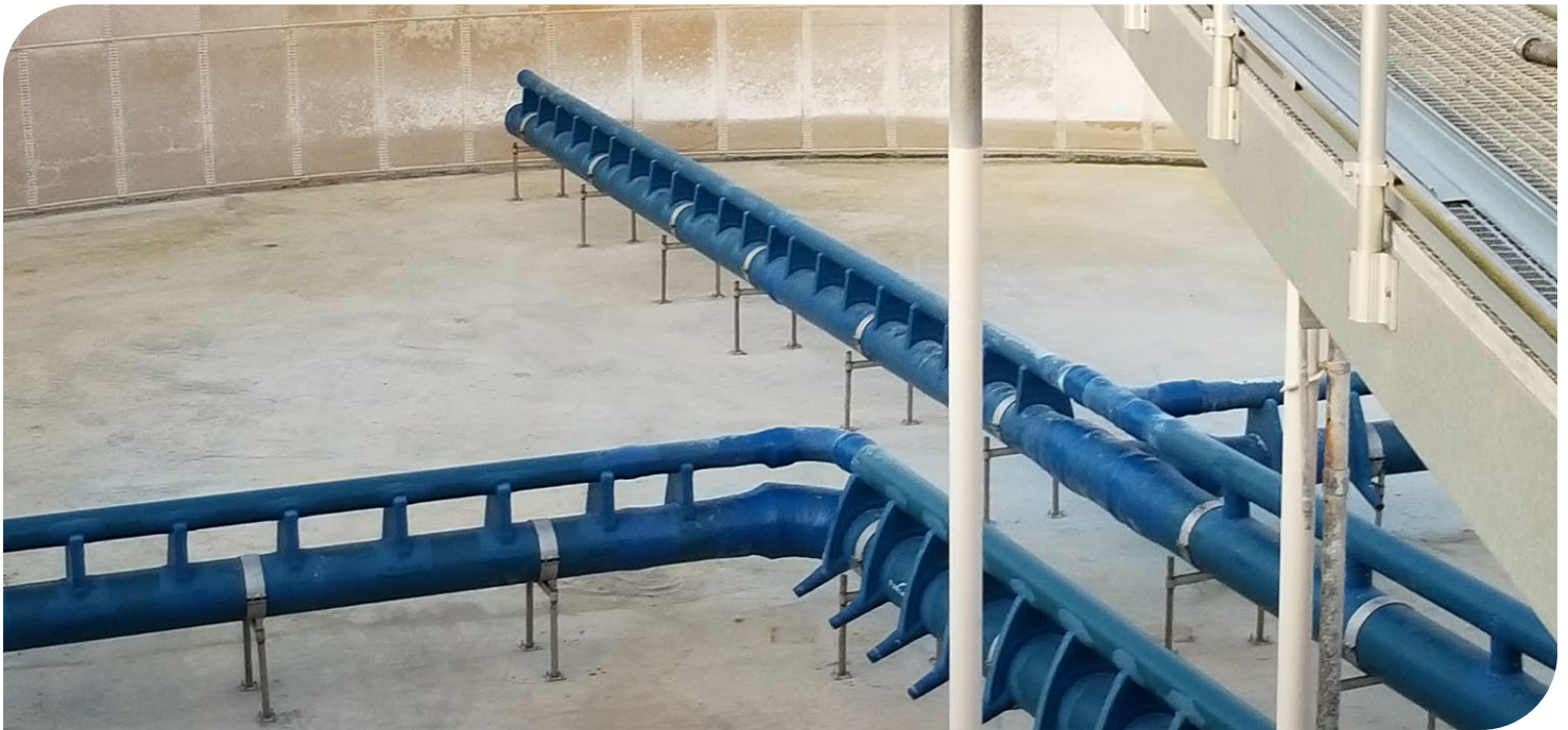
VariOx Jet Aeration system in nitrification basin
